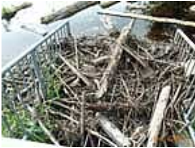
Beaver dam at the trash rack showing woody debris and mud.
