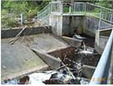
The upstream end of the fish ladder/outlet control structure.
